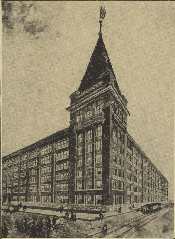
Figure 22. New buildings now nearing completion at the Western Electric Company's Hawthorne plant to be used for the manufacture of machine switching equipment.
