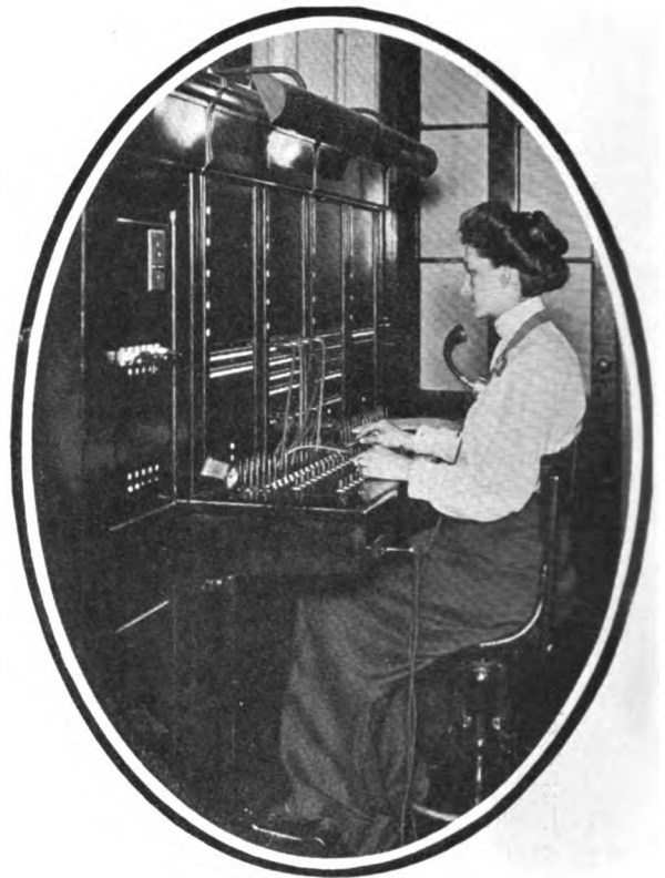
Most of the University's Telephones are Served From This Two Position Switchboard, Located on the Second Floor of College Hall. After 11 P. M. Certain Stations are Trunked Through to the "Baring" and "Preston" Central Offices.
