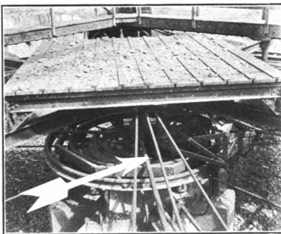
Detail of Sliding Contacts on Movable Crane (See description above upper illustration)
