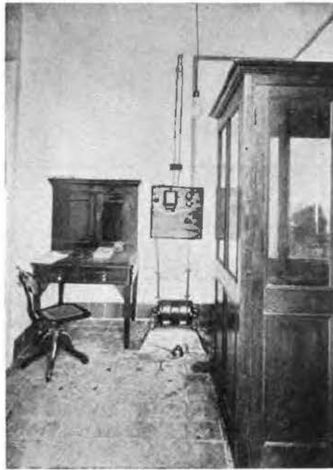
A Western Electric charging plant in the Central Telegraph Station at Matanzas
