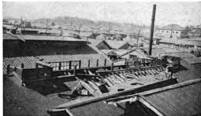
Another View of the Wrecked Roof of the Blacksmith Shop
