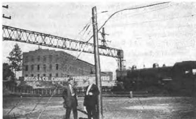
H. H. Shepard of the New Haven, and C. R. Wharton, Western Electric, inspecting the new cable
