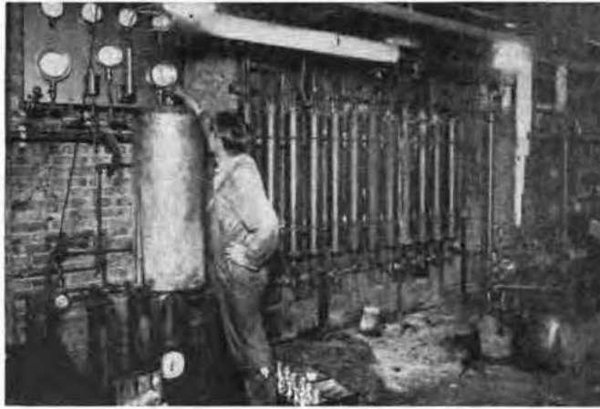
Liquid air machine recently installed for work on Government apparatus
