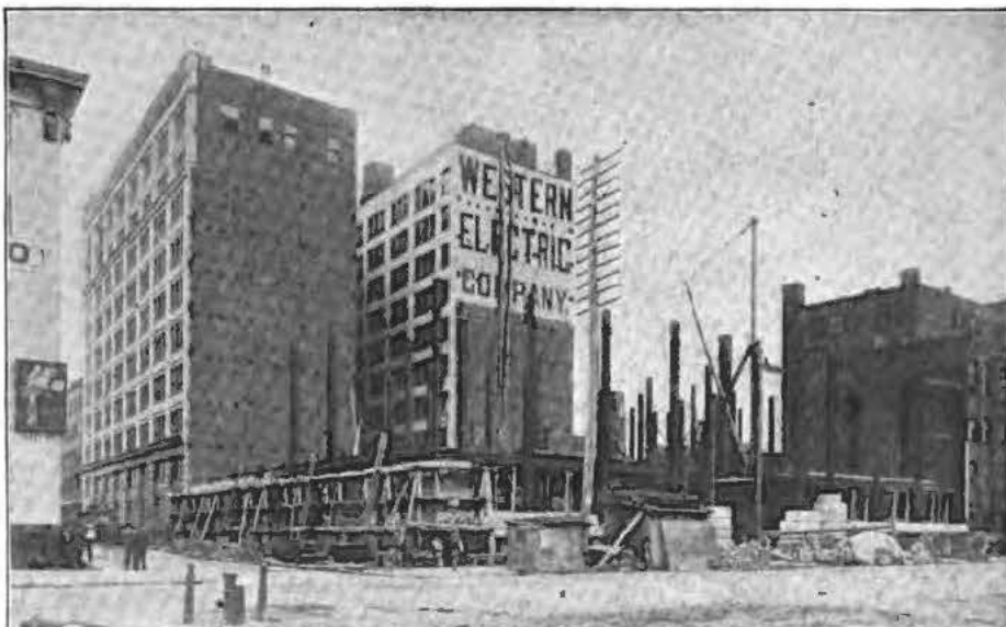
THE BEGINNINGS OF THE WEST STREET BUILDING Sections B and C as they looked in 1897. In the foreground, the foundations of Sections A and D
