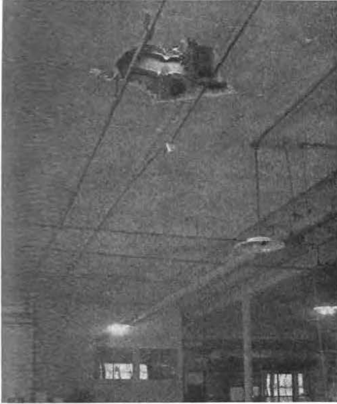
Hole in ceiling of shop office
