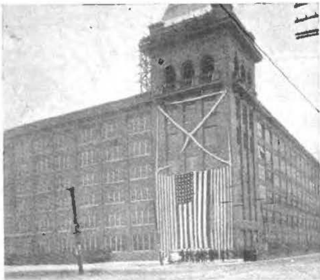
View of the Partially Completed Tower Group showing the Decorations in Place for the Corner-stone Ceremonies.
