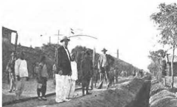
Mr. Rothe, Chief Engineer, Tientsin, and Mr. Carey inspecting duct runs, Tientsin
