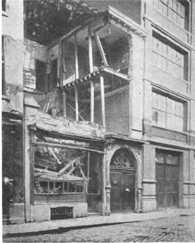
A Shot That Came Too Close for Comfort. The Building on the Right Is Part of the Antwerp Factory
