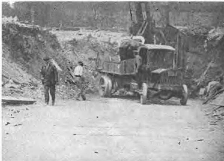
This shows the beginning of the gigantic process of removing 50,000 square yards of dirt to make way for the foundations of the 395 Hudson Street building
