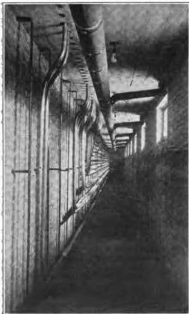
CABLE RUNWAY NEW STEWART OFFICE.
