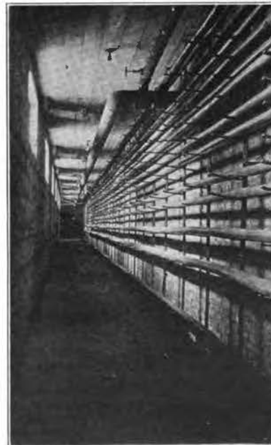
CABLE RUNWAY, NEW STEWART OFFICE.
