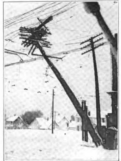
STORM CONDITIONS IN CLEVELAND. A Bad Tangle of Telephone and Trolley Wires.
