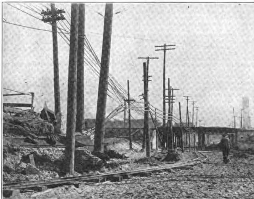
UNDERGROUND CABLE ON POLES ON SOUTH CHICAGO AVENUE, CHICAGO.
