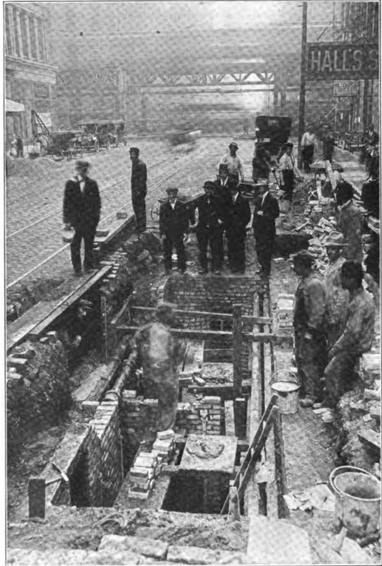
MAMMOTH CABLE VAULT ON WEST WASHINGTON STREET, CHICAGO. This picture gives a splendid idea of what underground work in a large city means.
