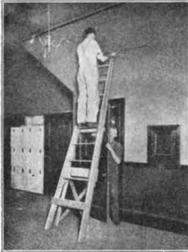
THE WRONG WAY.
