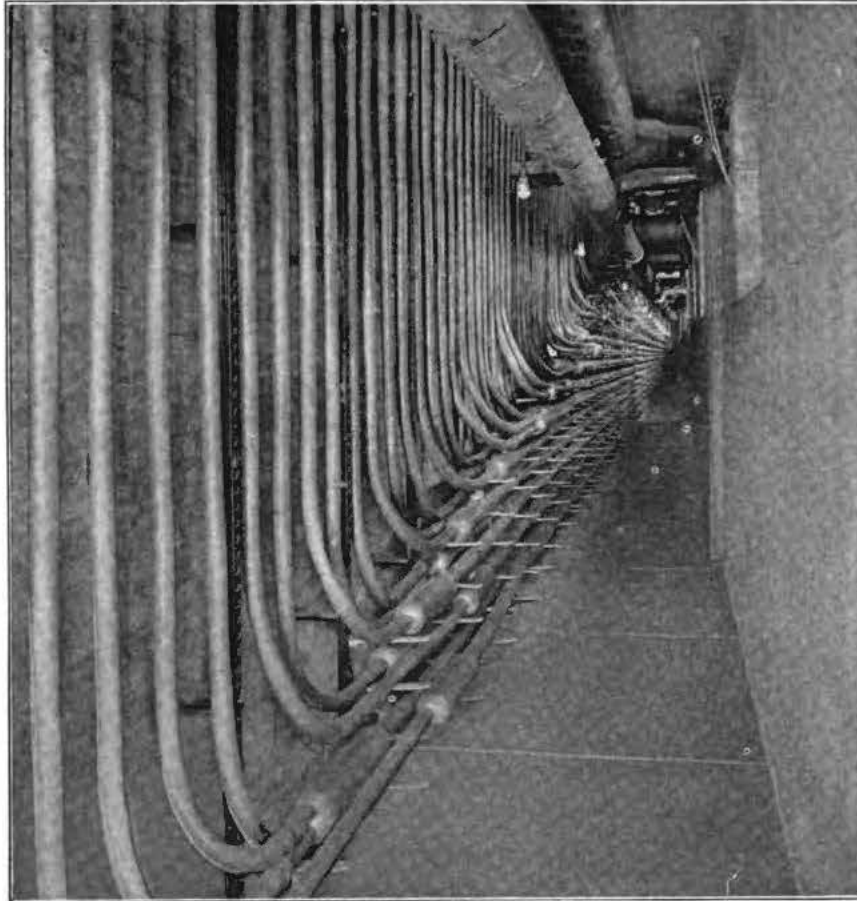
CABLE VAULT, NEW HYDE PARK OFFICE.
