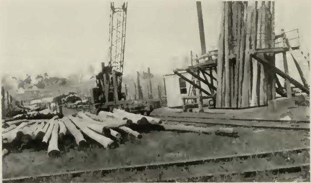
Fig. 20—Preparation Skids Opposite Treating Tanks in Nashville Yard
