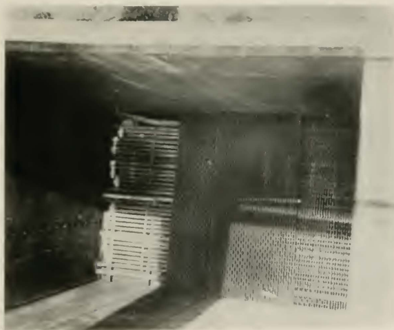
Fig. 27—Bottom of Treating Tank Showing Horizontal Radiators and Grids Covering Them
