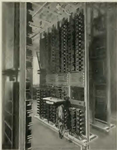
Fig. 6—Bank of 2-wire telephone repeaters
