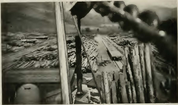
Fig. 5—Yard Layout at One End of Natural Bridge Yard, Viewed from Mast of Derrick
