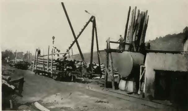
Fig. 15 - Stiff Leg Derrick Removing Poles from Treating Tank and Loading Them on Flat Car
