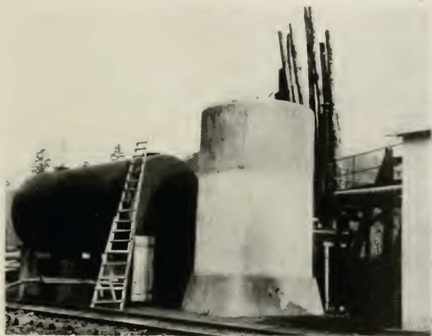
Fig. 29—Vertical Hot Oil Tank with Insulated Covering
