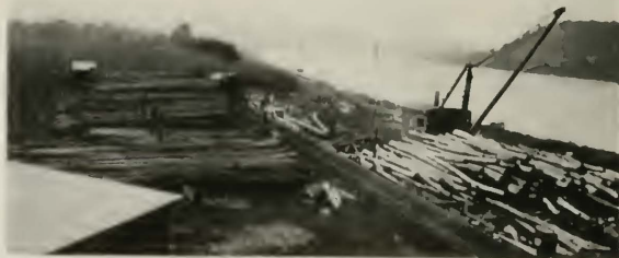
Fig. 12—Derrick for Handling Poles from River Rafts to Piles or Pole Cars in the Yard
