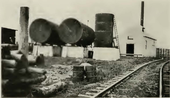
Fig. 28—Horizontal Cold Oil Tanks and Vertical Hot Oil Tank
