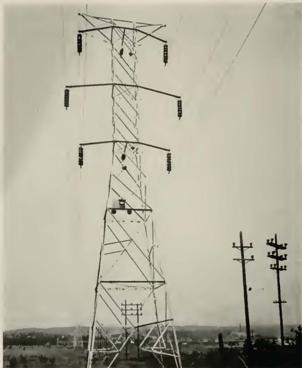
Fig. 16 Distant End of Typical Coupling Wire Installation Showing Coupling Wire Tuning Unit
