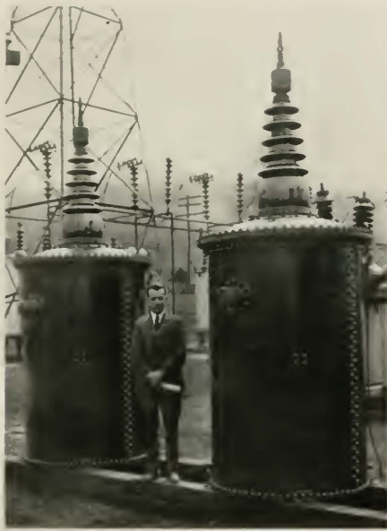
Fig. 13—110 K.V. Coupling Condensers Used for Coupling Carrier Circuit to a 110 K.V. Power Line
