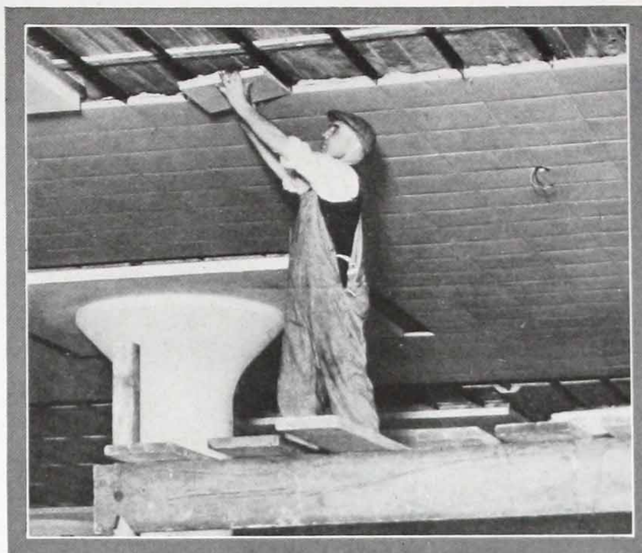
This photograph shows J-M Sanacoustic Tile being applied. Metal lath and plaster has been eliminated as unnecessary wherever this acoustical treatment is used. J-M Sanacoustic Tile is easy to install, yet makes a permanent, fire-proof job
